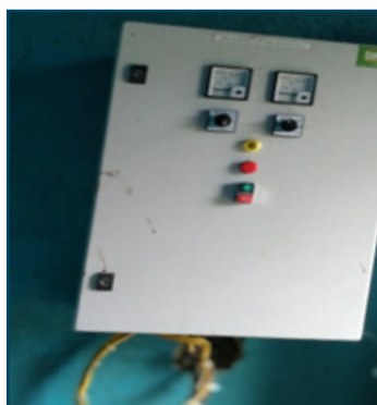
Foto No. 2 Interruptor Principal
